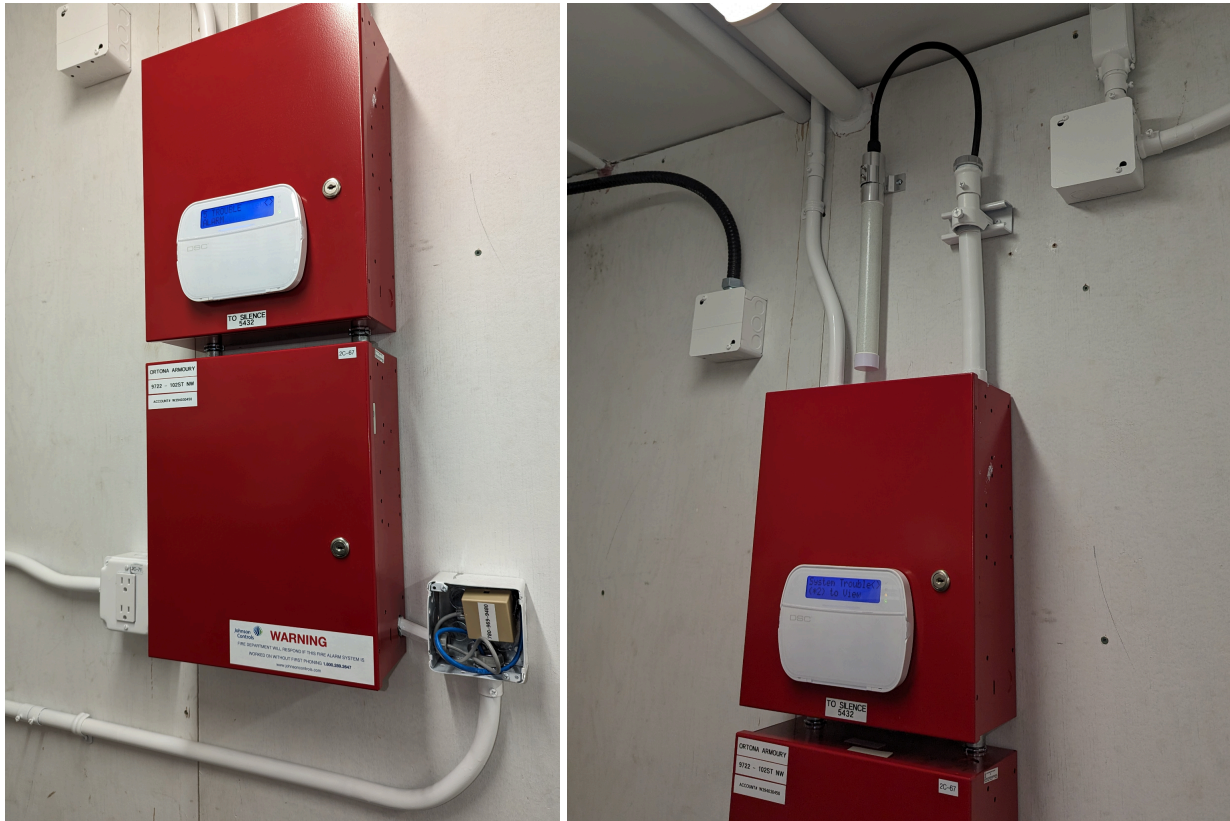
DSC H32-612TLLEC Fire Monitoring Typical Installation Photo
