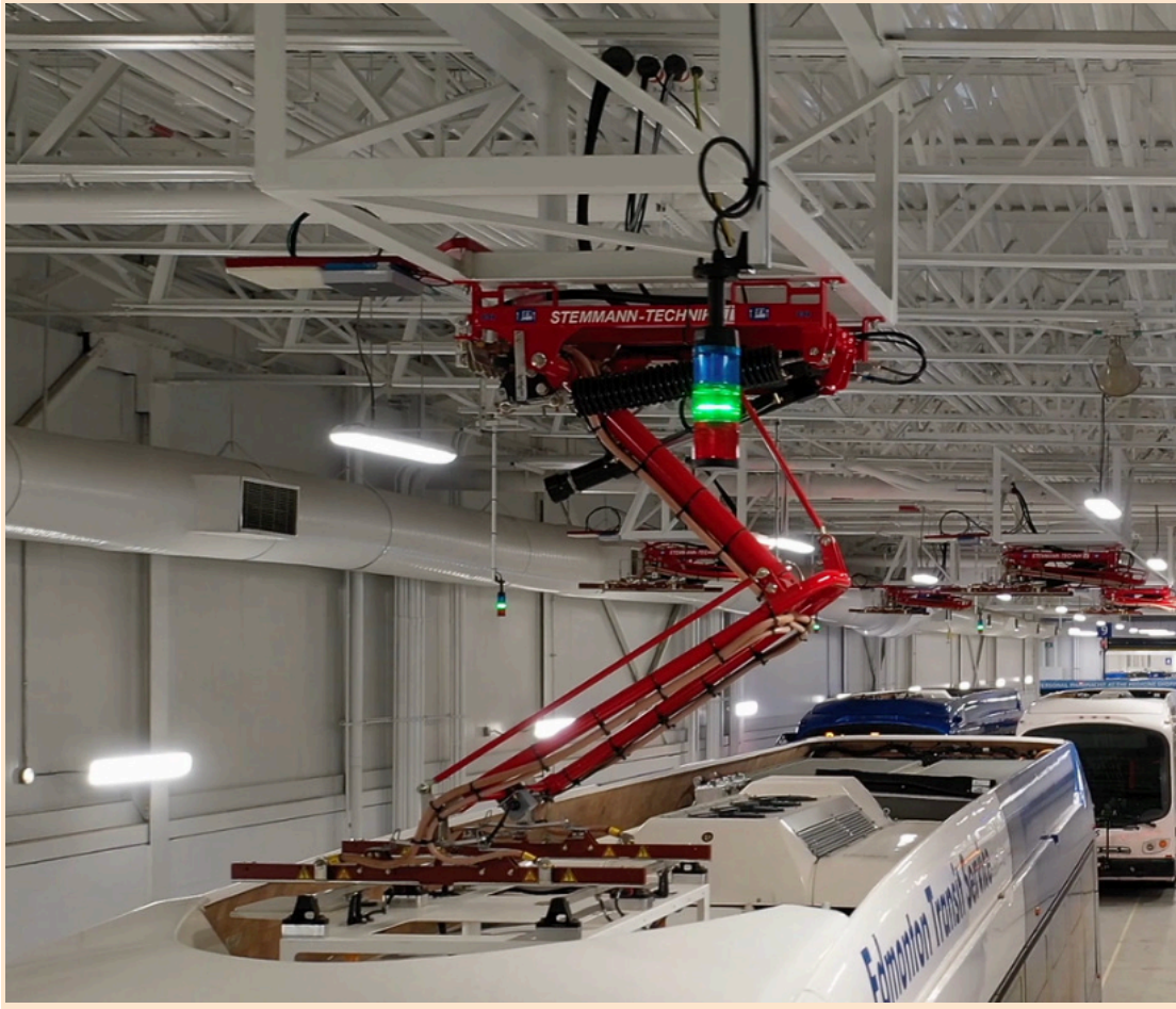
Figure I4: Katleen Andrew Garage Example (Stemmann Technik “Charging Panto”)
